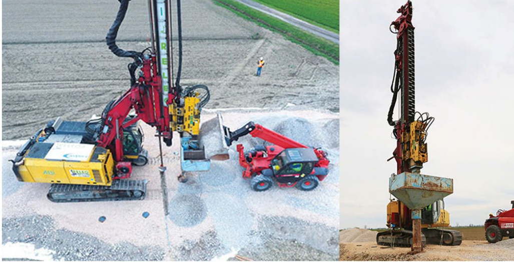
Figure 5.1: (Left) Aerial photograph at the Bondeno test site showing the track mounted ramming hammer with a hopper being loaded with gravel aggregate. (Right) Photo of a typical hopper and mandrel being compacted by the vibratory power unit ( http://www.releo.it/blast-test-impact-pier.php ).
