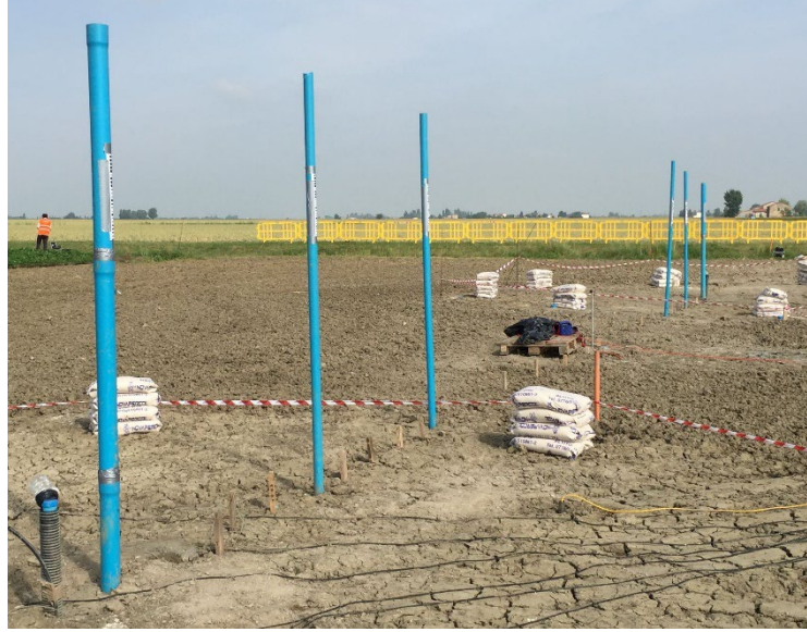
Figure 6.6: Oblique view of the six blue PVC surface settlement rods, and the sixty-two surface settlements stakes, across the test field.
