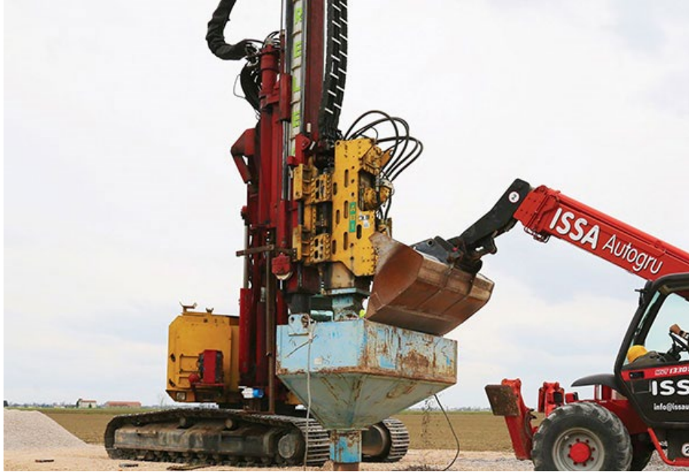
Figure 3.3: A typical RAP vibratory power unit with hopper being loaded with granular backfill ( http://www.releo.it/blast-test-impact-pier.php ).
